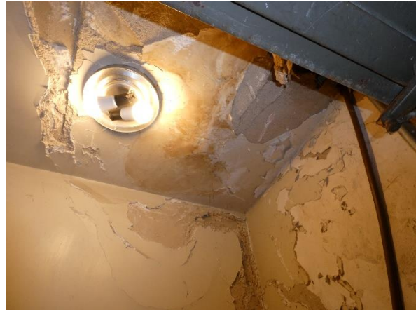
Photo 110 - Garage: Damaged ceiling and wall finishes.
