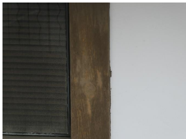
Photo 54 - Building 340: Condition of painted wood trim.
