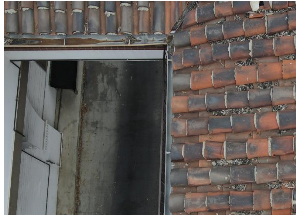
Photo 74 - Building 320: Condition of gutter system at the roof perimeter.
