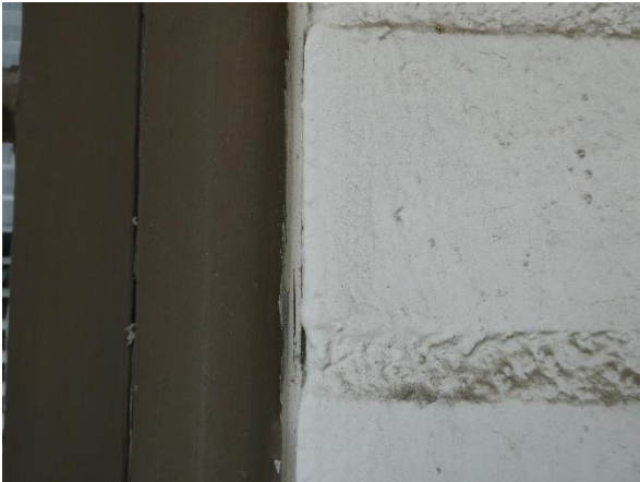
Photo 61 - Building 340: Sealant at window penetrations is deteriorated.
