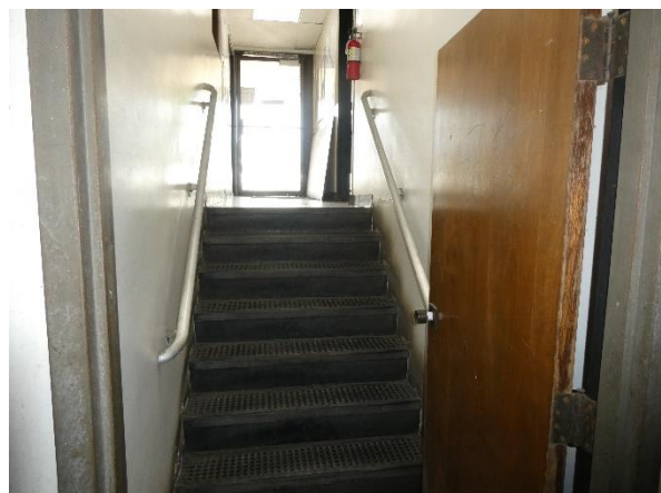
Photo 96 - Building 320: Interior stair finishes from the parking garage to the Maintenance Department.
