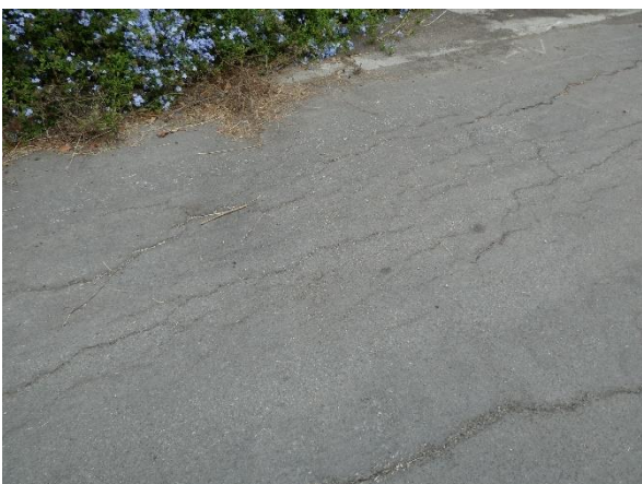
Photo 5 - Remote Lot: Cracks at drive lanes.
