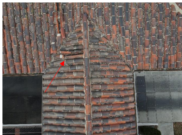
Photo 78 - Delaminated terracotta tiles at walkway roof.
