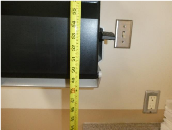
Photo 169 - Building 320 (Homeowners Association): Paper towel dispenser lever is in excess of 48-inches AFF.
