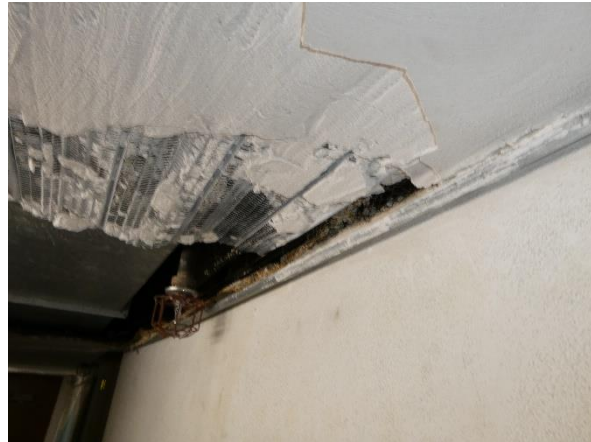
Photo 104 - Building 320: Damaged corridor plaster ceiling finishes.
