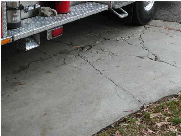
Photo 19 - Damaged concrete apron.
