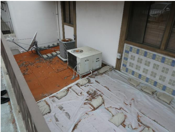
Photo 87 - Building 340: Condition of modified bitumen roof systems at the South building elevation.
