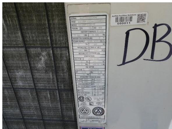
Photo 138 - Building 340: Corroded condenser unit coil fins.
