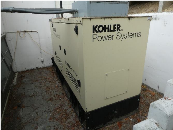
Photo 151 - Building 340: Kohler 80KW standby generator.
