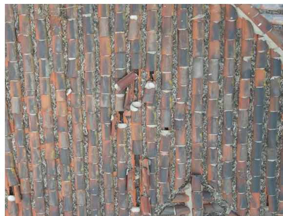
Photo 83 - Building 340: Missing fasteners at select steel components.
