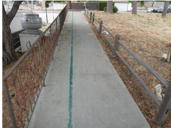
Photo 164 - Building 340: Excess slope, non-compliant guardrail, and intermediate landings not provided at the site ramp.
