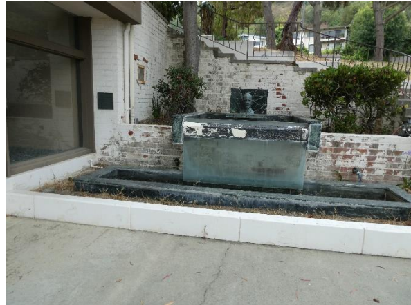
Photo 26 - Non-functioning water feature.
