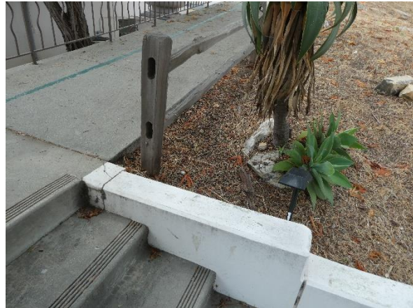
Photo 20 - Handrails not provided at the site stairs.
