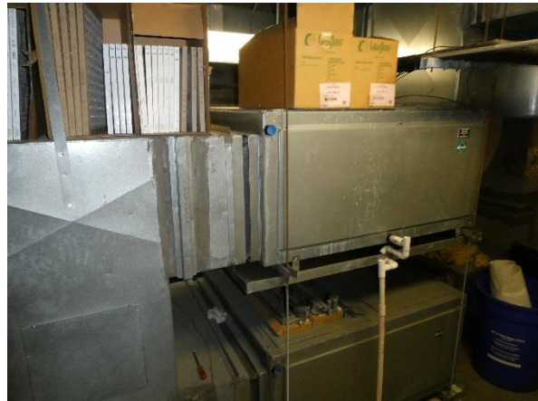
Photo 142 - Building 340: Fan/coil units located in the basement.
