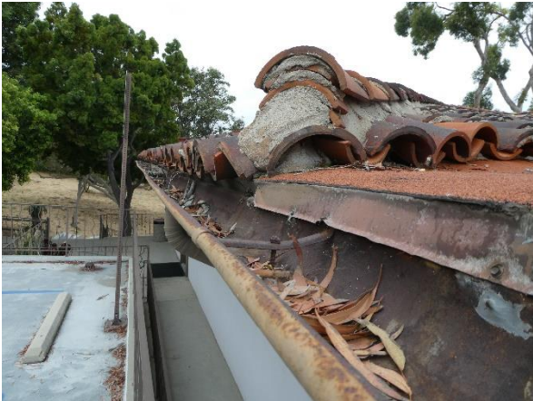
Photo 85 - Building 340: Condition of metal gutters.
