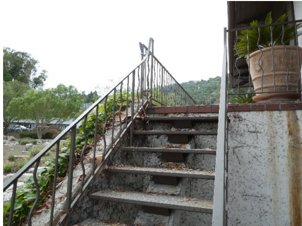
Photo 38 - Building 320: Open risers and excessive baluster spacing at the building stairs. Note: Guardrail not provided.
