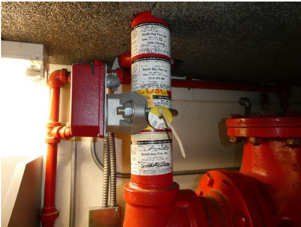
Photo 159 - Building 340: Main fire riser.
