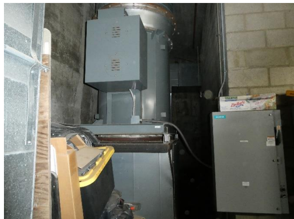
Photo 144 - Garage: East ventilation fan.
