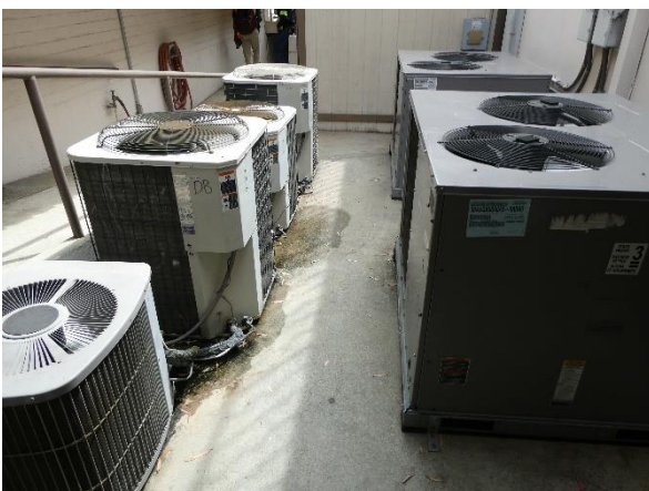
Photo 137 - Building 340: Pad-mounted condensing units.
