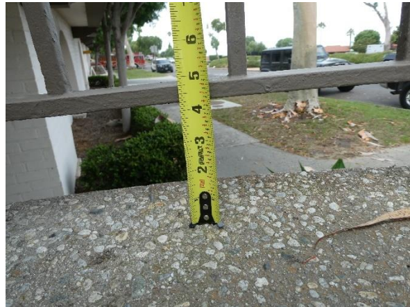
Photo 46 - Building 320: The bottom of the guardrail to the finish floor exceeds 4 inches.
