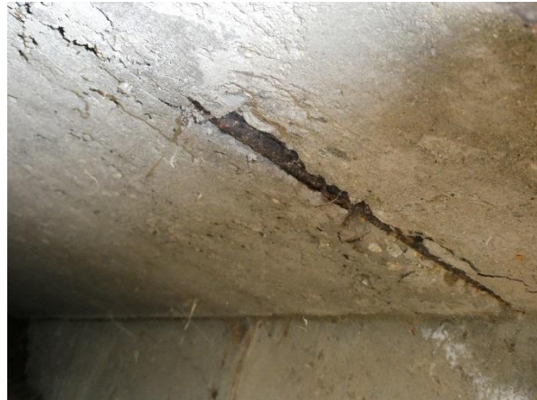
Photo 14 - Exposed rebar at the underside of the site ramp.
