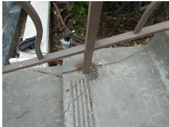
Photo 22 - Cracked concrete at guardrail post anchors.
