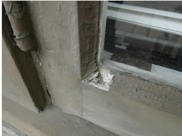
Photo 62 - Building 340: Glazing putty at select windows is missing.
