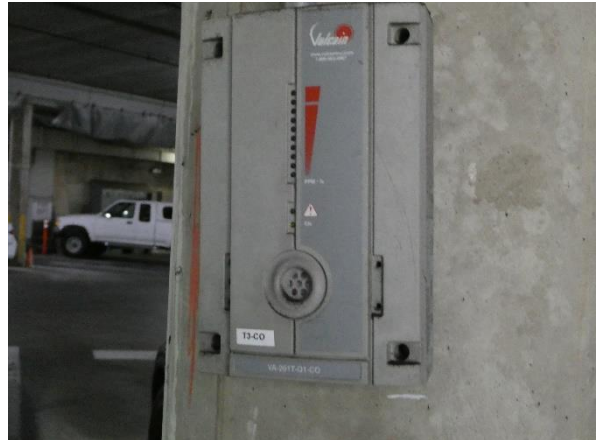
Photo 146 - Garage: Column mounted carbon monoxide sensor.
