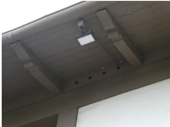
Photo 64 - Building 340: Damaged wood trim and overhang.
