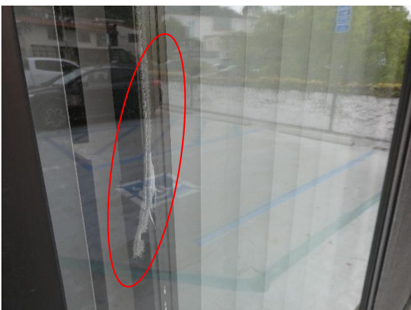
Photo 35 - Building 320: Damaged weatherstripping at window.
