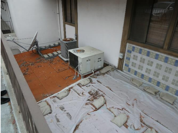
Photo 139 - Building 340: Roof-mounted condensing units.
