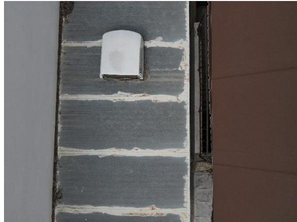
Photo 76 - Corroded sheet metal at the freestanding building adjacent to Building 340.
