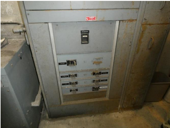
Photo 147 - Building 320: Sylvania main switchgear.
