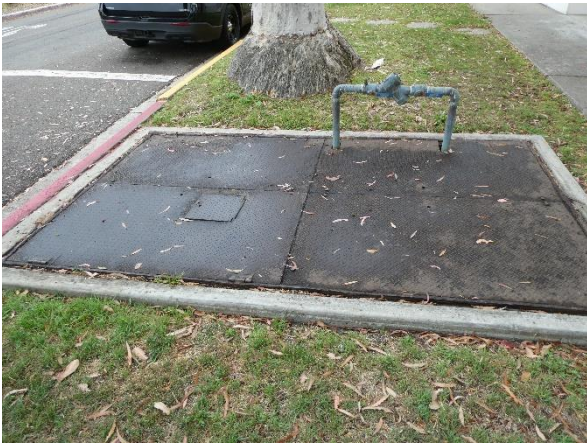
Photo 153 - Building 340: Domestic water backflow preventer.
