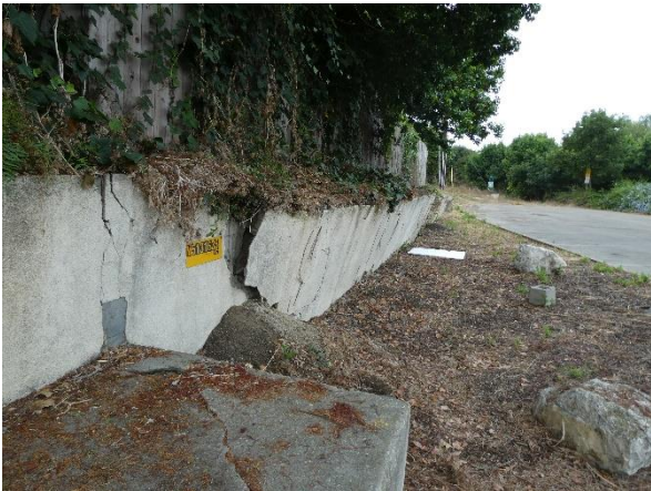
Photo 9 - Rotation and retaining wall failure near the southwest site boundary.
