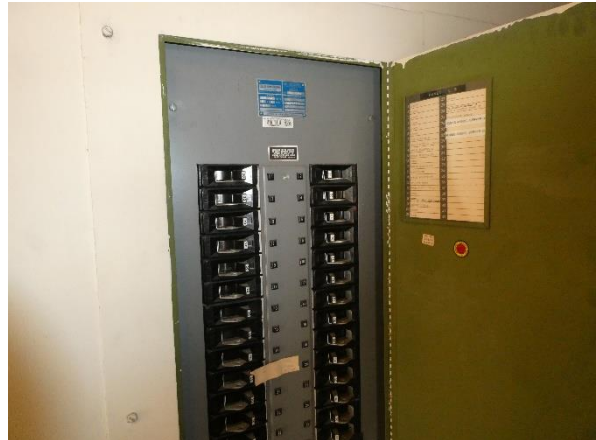
Photo 152 - Building 320: Electrical distribution panel.
