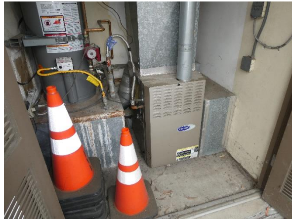
Photo 136 - Building 320: Newer furnace installed in 2 nd floor mechanical room.
