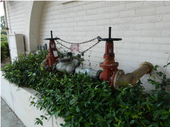
Photo 157 - Building 320: Fire water backflow preventer.
