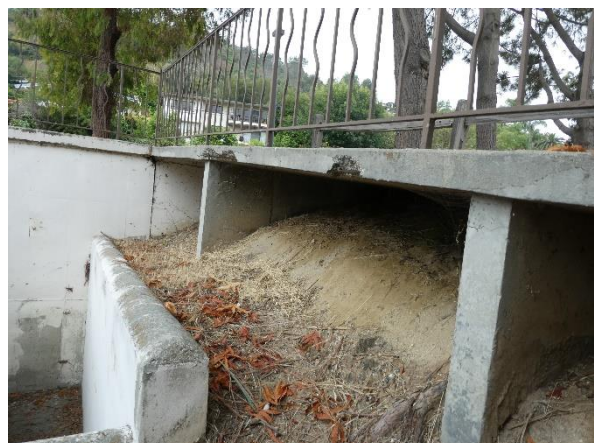
Photo 12 - Damaged concrete ramp and erosion at the under-ramp locations.
