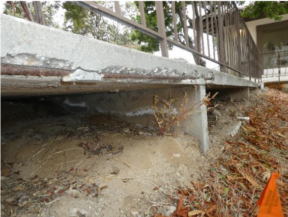
Photo 13 - Exposed rebar and spalled concrete at the site ramp.
