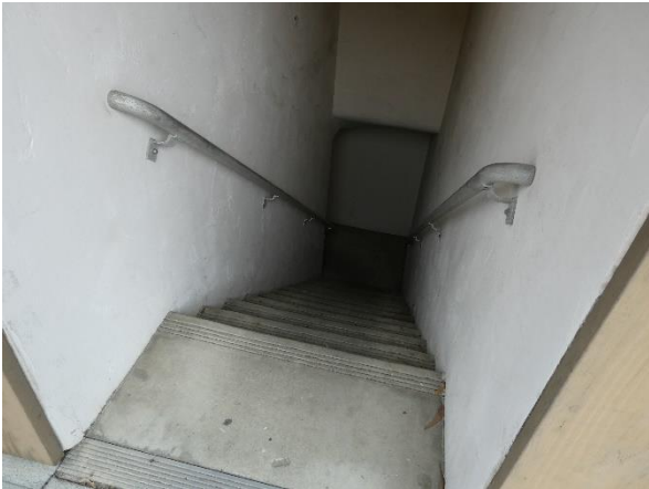
Photo 37 - Building 320: Handrail extensions not provided at the building exterior stair.
