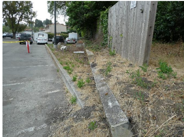
Photo 10 - Retaining wall rotation near the southwest site boundary.
