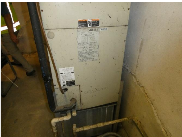
Photo 143 - Building 340: Older fan/coil units located in the basement.
