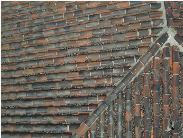
Photo 73 - Building 320: Multiple cracks in mortar joints at clay tile intersections.
