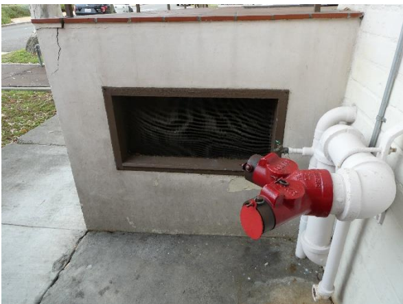
Photo 161 - Building 340: Fire department connector.
