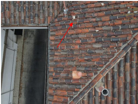
Photo 71 - Building 320: Delaminated terracotta tile throughout the field of the roof.
