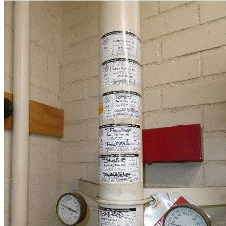
Photo 158 - Building 320: Main fire riser.
