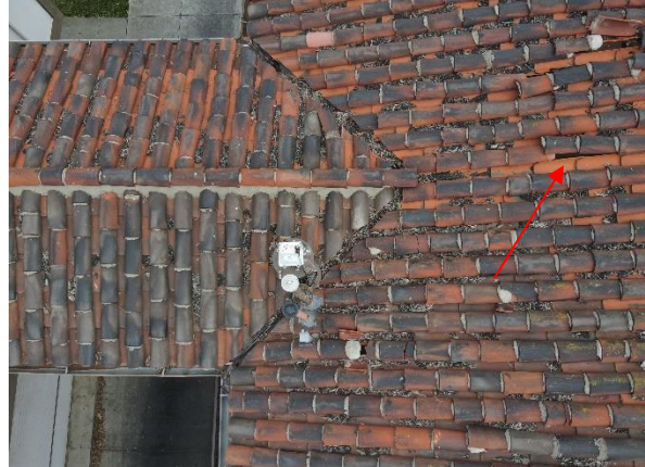
Photo 72 - Building 320: Exposed roof underlayment.
