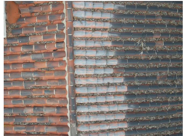
Photo 82 - Building 340: Discolored terracotta tiles at the field of the roof.
