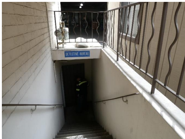
Photo 66 - Building 340 (Detective Bureau): Handrail extensions not provided at the stairs.
