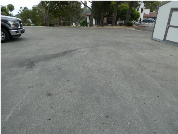
Photo 1 - Remote Lot: Condition of the asphaltic concrete pavement.
