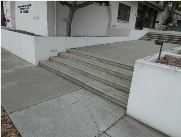
Photo 25 - End and intermediate handrails not provided at site stairs.
