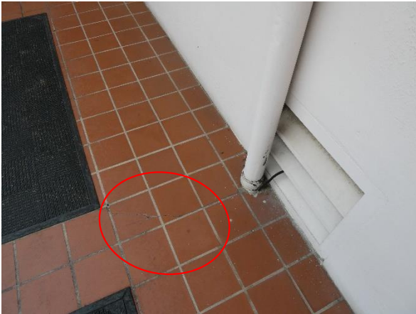
Photo 43 - Elevated walkway: Cracked flooring.
