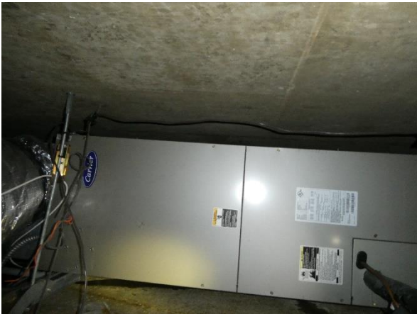
Photo 141 - Building 340: Fan/coil units mounted above suspended ceiling.
