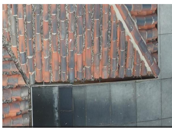
Photo 84 - Building 340: Condition of the gutter system at the roof perimeter.
