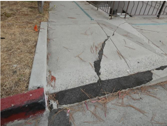
Photo 15 - Concrete repair needed at the ramp landing.
