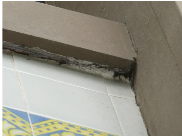
Photo 34 - Building 320: Deteriorated sealant.
