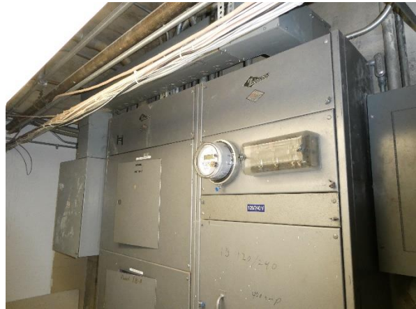
Photo 148 - Building 340: Zinsco combination main switchgear.
