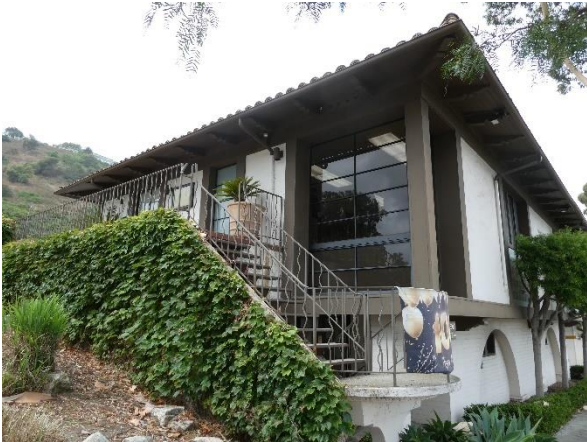
Photo 31 - Building 320: East elevation. Note: Guardrail not provided.
