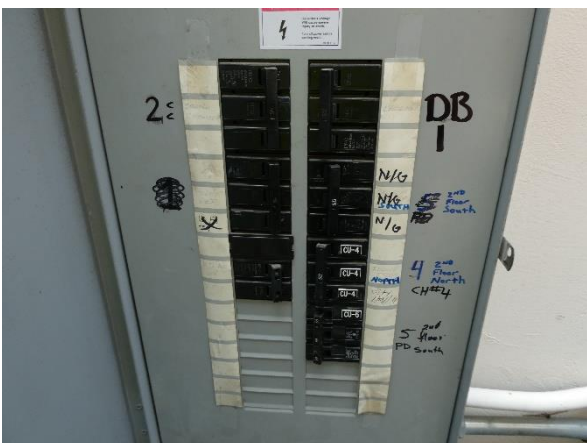
Photo 149 - Building 340: Three-phase panel located outdoor near the condensing units.
