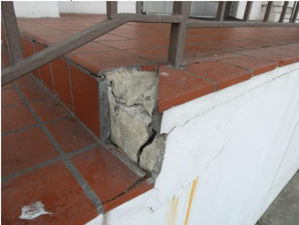
Photo 69 - Building 340 (Police Department): Damaged tile and concrete at guardrail post anchor.
