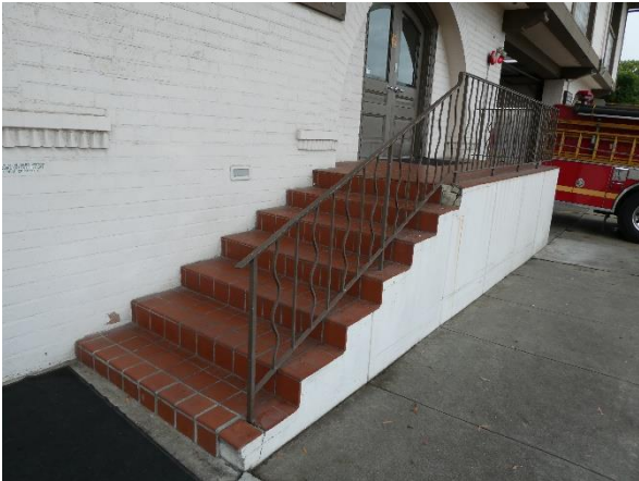
Photo 67 - Building 340 (Police Department): Handrail provided at one side, and handrail extensions not provided at the exterior stair.
