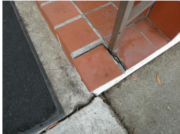
Photo 68 - Building 340 (Police Department): Damaged tile at guardrail post anchor.
