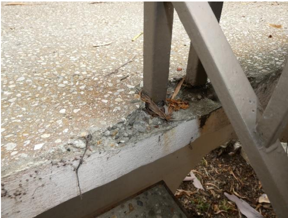
Photo 45 - Building 320: Spalled concrete at guardrail post anchor.
