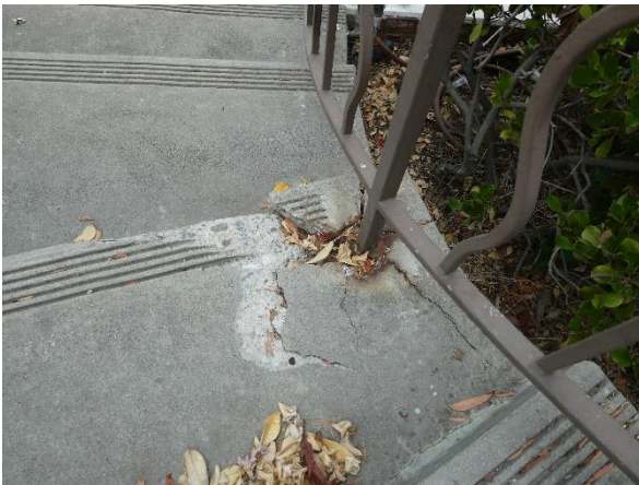
Photo 21 - Spalled concrete at guardrail post anchors.
