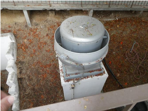
Photo 145 - Garage: West ventilation fan.
