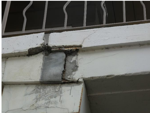
Photo 40 - Spalled concrete at the elevated walkway.
