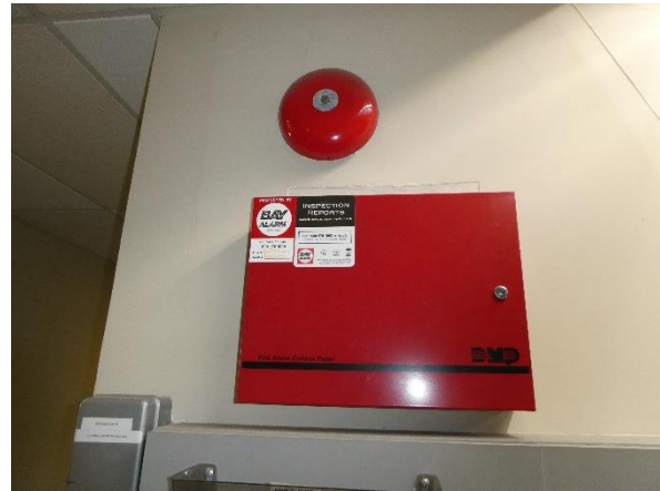
Photo 160 - Building 340: Fire alarm control panel and alarm bell.
