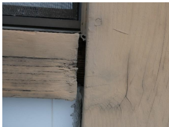
Photo 36 - Building 320: Condition of painted wood trim and missing joint sealant.
