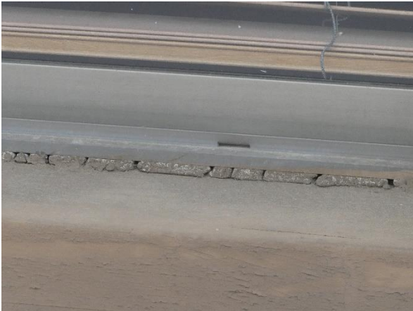
Photo 55 - Building 340: Deteriorated grout between the window frame and wood trim.
