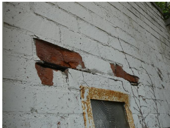
Photo 24 - Select finishes at the masonry veneer retaining wall are spalled, and painted finishes are peeled.
