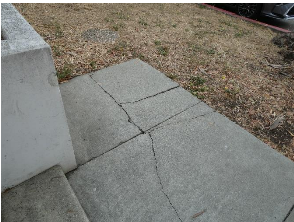
Photo 17 - Missing handrail and cracked concrete pavement near the cast-in-place site stairs adjacent to Building 340.
