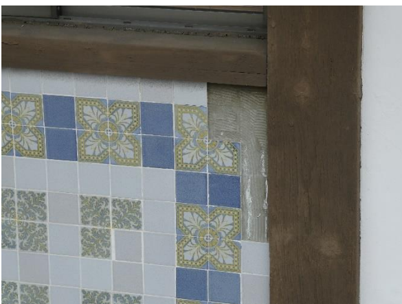
Photo 53 - Building 340: Missing ceramic tiles.
