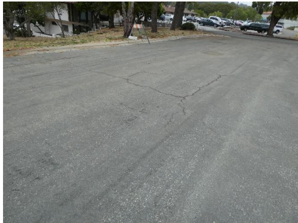
Photo 4 - Remote Lot: Cracks at drive lanes.
