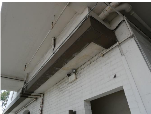
Photo 41 - Elevated walkway: Evidence of water intrusion.
