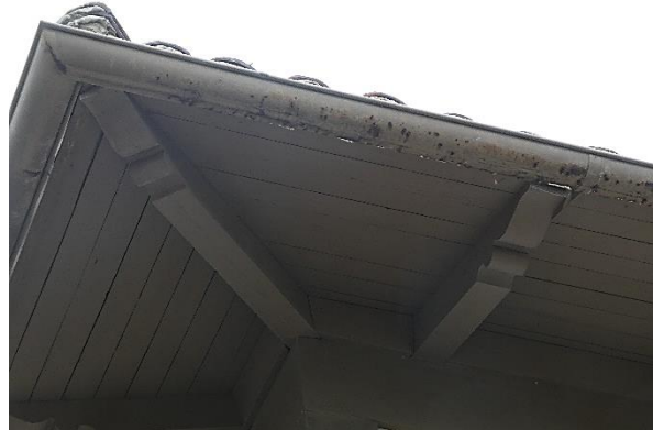
Photo 86 - Building 340: Gutter penetrations at the North elevation.
