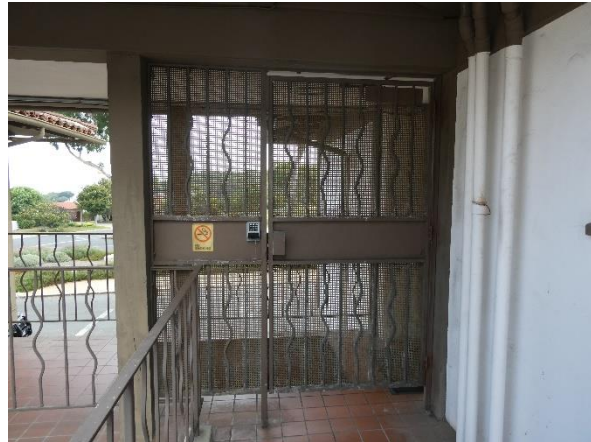
Photo 44 - Elevated walkway: Painted finishes are deteriorated and corroded at the access door.
