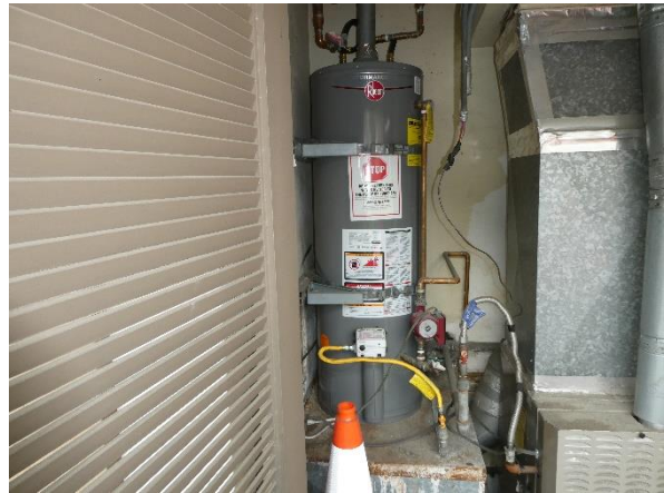
Photo 154 - Building 320: Domestic water heater.
