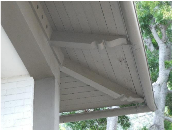
Photo 63 - Building 340: Damaged wood trim at overhang.
