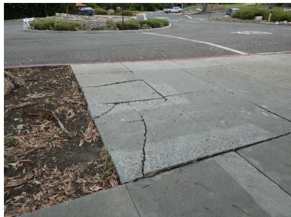
Photo 18 - Cracked and uneven concrete-paved walking surfaces near the north site boundary.
