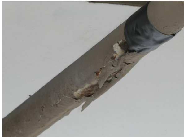
Photo 56 - Building 340: Select painted metal surfaces are peeled.
