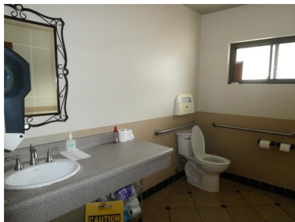
Photo 168 - Building 320 (Homeowners Association): The bottom edge of the reflective surface exceeds 40-inches AFF.
