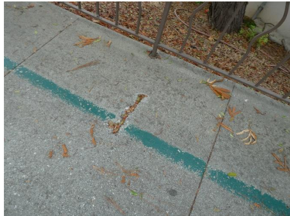
Photo 16 - Damaged concrete at the site ramp.
