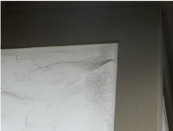
Photo 33 - Building 320: Soiled painted finishes.
