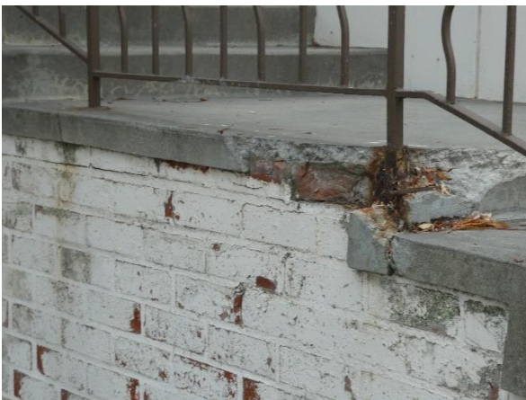
Photo 23 - Spalled concrete at guardrail post anchors.
