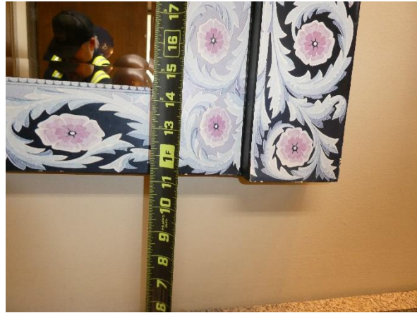
Photo 170 - Building 340 (City Hall): The bottom edge of the reflective surface exceeds 40-inches AFF.
