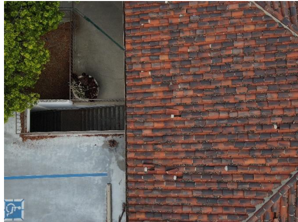
Photo 80 - Building 340: Delaminated terracotta tiles throughout the field of the roof.
