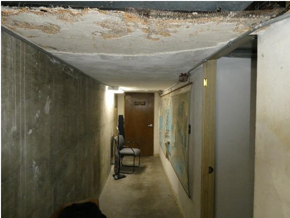
Photo 103 - Building 320: Damaged corridor plaster ceiling finishes.
