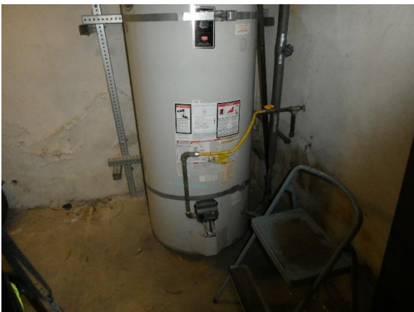
Photo 155 - Building 340: Domestic water heater.
