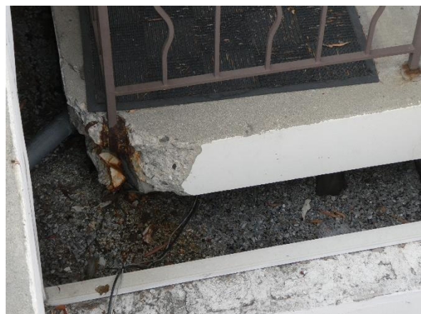
Photo 60 - Building 340: Damaged walkway concrete pavement near City Hall 2022
