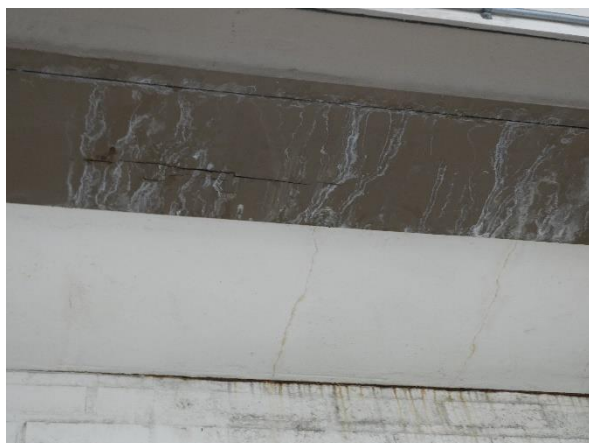
Photo 42 - Close-up of staining and damaged wood trim from the previous photo.
