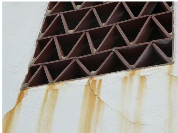
Photo 58 - Building 340: Surface stains and cracking at the tower.
