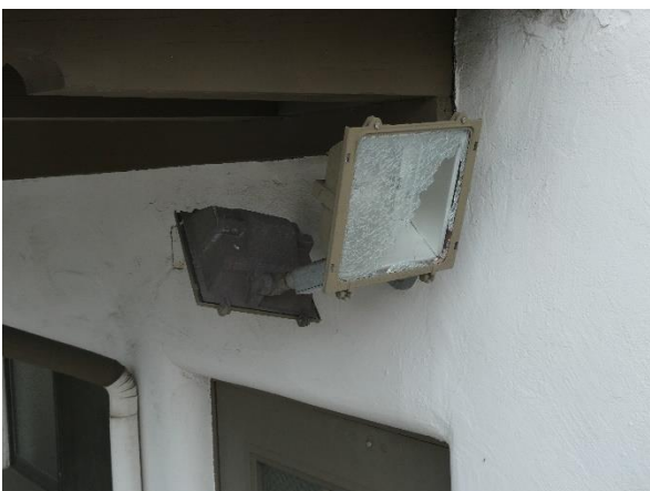
Photo 59 - Building 340: Damage surface-mounted lighting.
