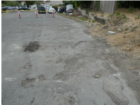
Photo 2 - Remote Lot: Select areas of the asphaltic concrete pavement are raveled.
